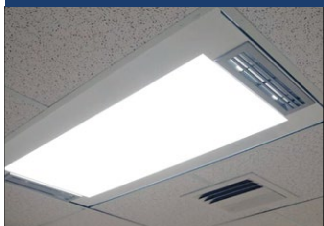
FIGURE 2. UV-C unit installed
